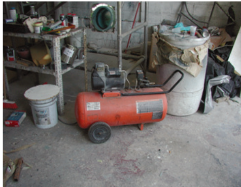
A compressor is a typical example of a noise source
