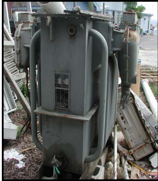
..... An out-of-use transformer
